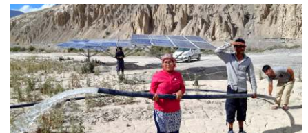
7.5 Hp Solar Irrigation Project (Spiti Valley)
